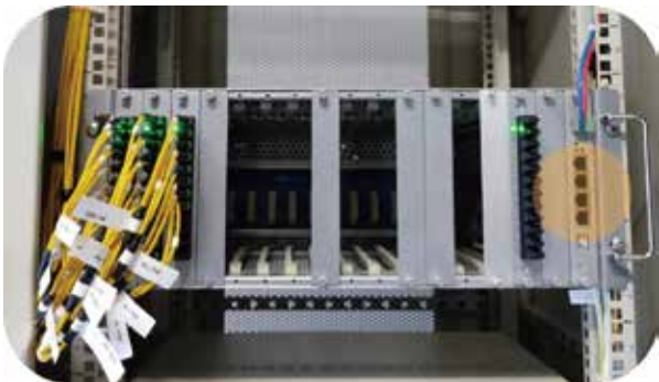
4U Monitoring Controlling Unit
